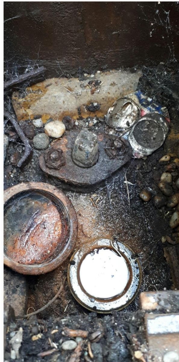
01452 – leaking hydrant valve Estimated 0.1 l/m
