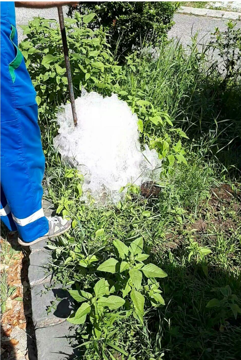
01411 – leaking hydrant valve Estimated 30 l/m
